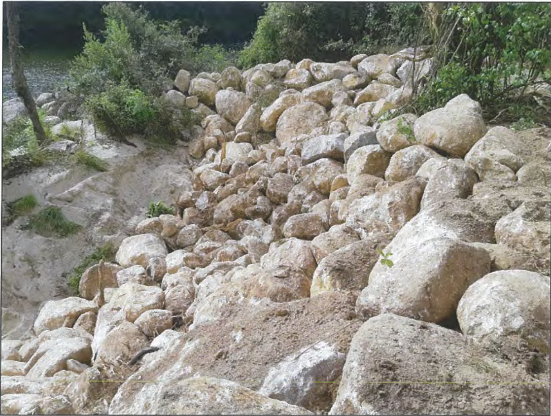
Rock protection at Spur #12, looking downstream.
