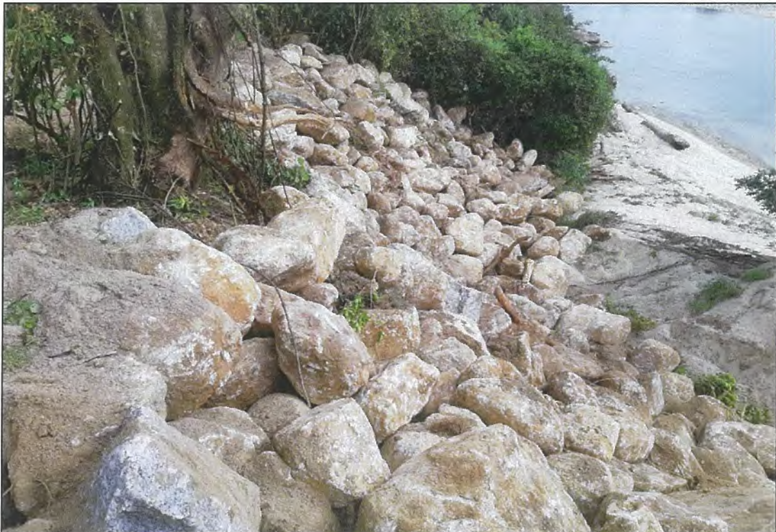
Rock protection at Spur #12, looking downstream.
